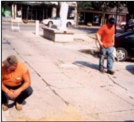
Testing new pavement repair materials behind statue of George Bartholomew on Court Street in Bellefontaine, OH
